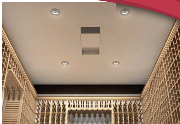
* Front grille and mounting bracket have been painted to match the ceiling
